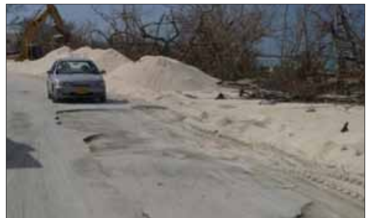
Hurricane Ivan storm surge removed part of the asphalt on West Bay Road north of Public Beach.
